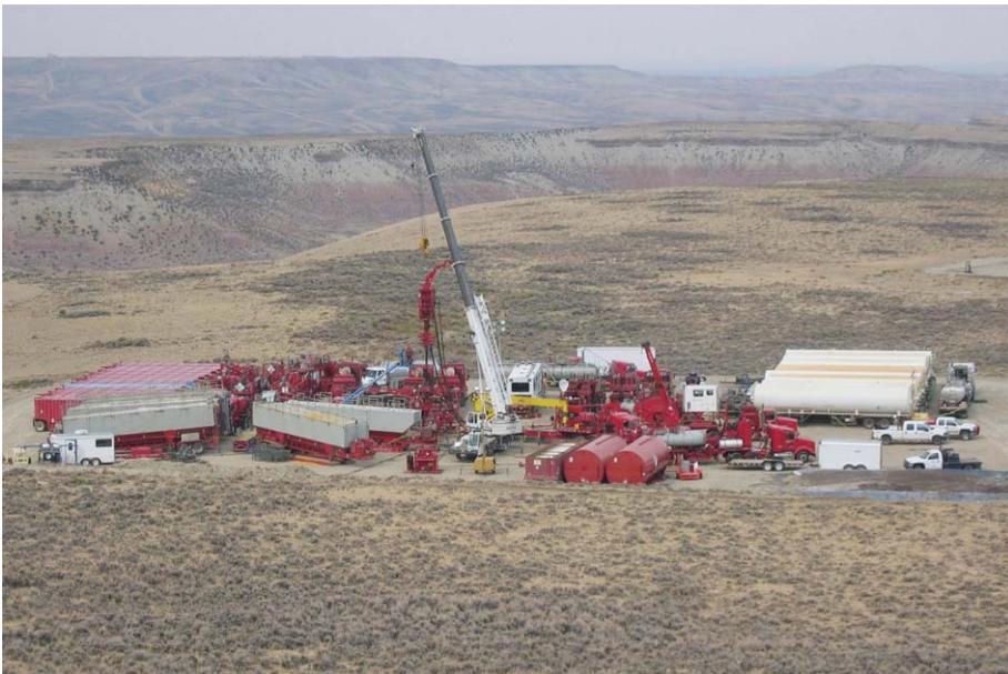
Figure 2.77 Pumping layout for large stimulation treatment, Wyoming, United States (photograph courtesy Michael C. Romer, ExxonMobil).
