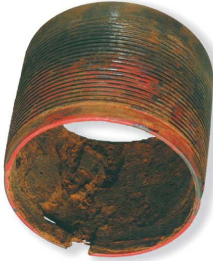
Figure 8.12 Corroded water injection carbon steel tubing.
