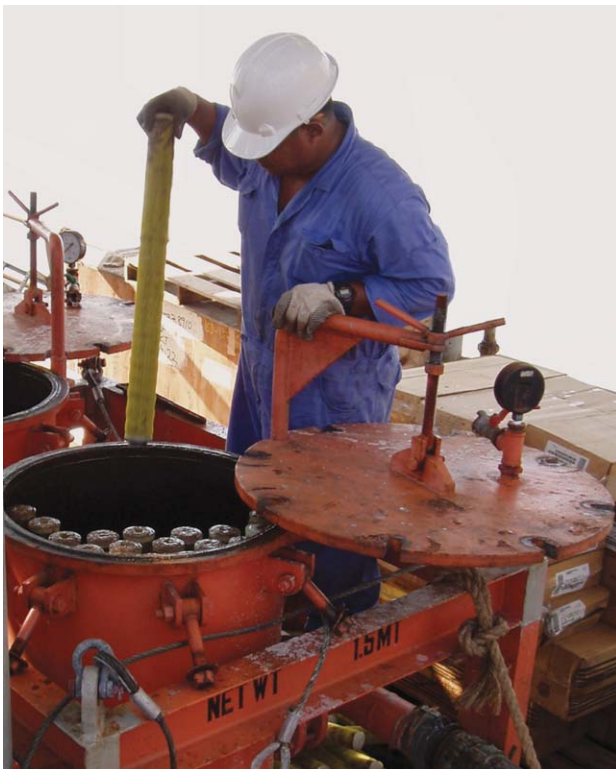
Figure 11.15 Replacing cartridges in a dual pod cartridge filter (photograph courtesy of Howard Crumpton).
