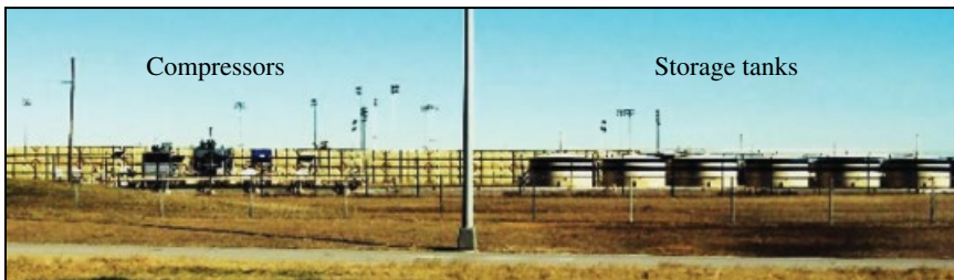
FIGURE 14.11 Surface equipment at a shale gas well pad.
