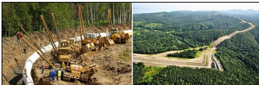
FIGURE 15.11 TransSakhalin pipeline system. (Source: Courtesy of Sakhalin Energy (2016), personal communication.)
