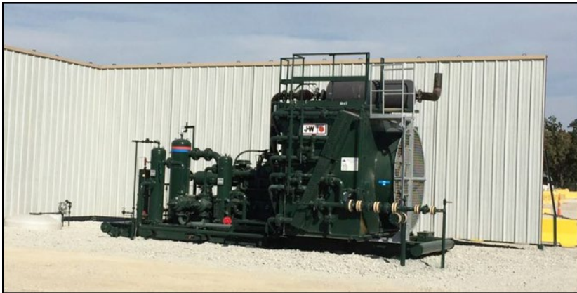
FIGURE 15.2 Gas compressor. (Source: © energy.fanchi.com (2015).)
